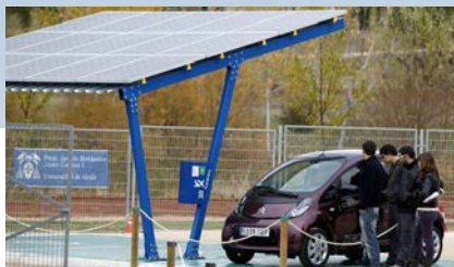
Location : Spain Rated system size: 2.85kW Construction type: Carport Completion date: 2011 Operator/installer: Sendekia
