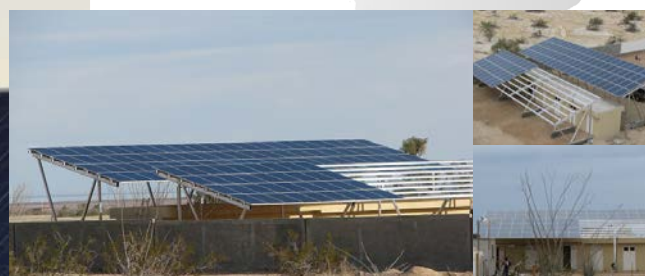
Location: Mexico Rated system size: 28.8kW Construction type: Carport Completion date: 2012 Operator/installer: Voltaika
